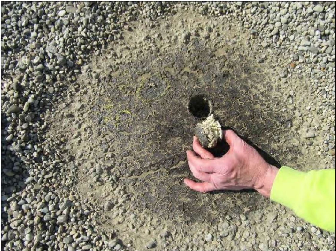
PHOTO #16: Core Cut #8 – View of roof core material 1/2" BUR, 1/2" perlite board, 2" ISO insulation board.
