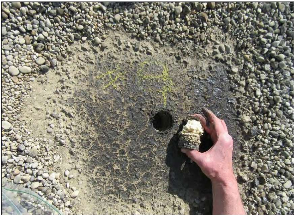
PHOTO #18: Core Cut #9 – View of roof core material 3/4" BUR, 1/2" perlite board, 2" ISO insulation board.
