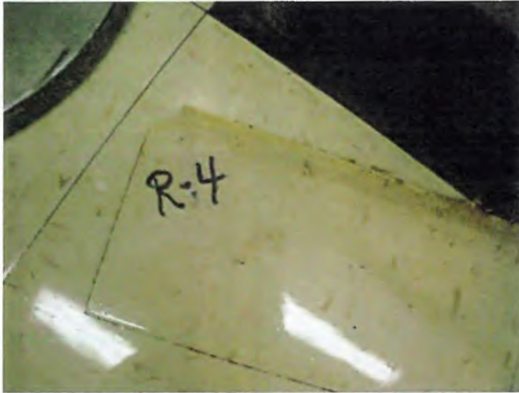
Photo 5: Off-White Floor Tile (R-4) Clinic. 3% Chrysotile Asbestos Detected (1.75% Point Count). Off-White Floor Tile Mastic, 7% Chrysotile Asbestos Detected.
