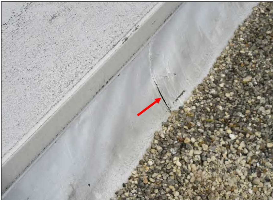
PHOTO #36: View of delaminating parapet wall flashing with an open/split membrane seam (Arrow).
