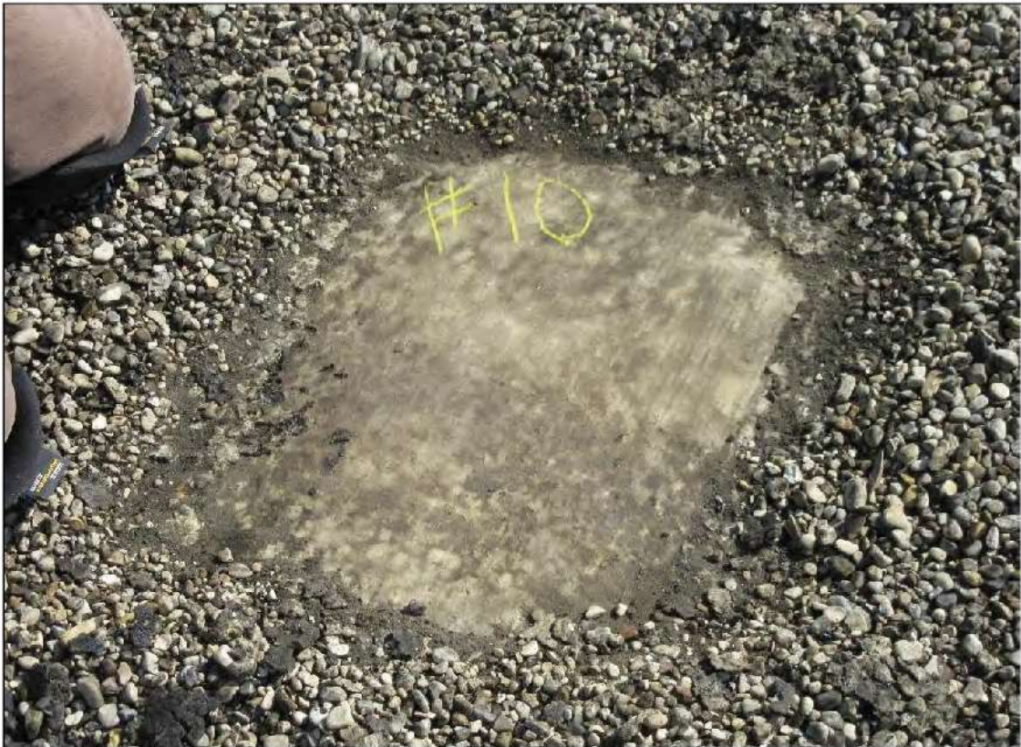
PHOTO #19: Core Cut #10 – View of Core Cut #10 located in the field of the roof between two roof drains. All material found in this roof core were WET.
