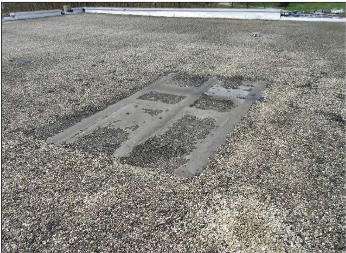
PHOTO #30: View of large repair patch installed near the west end of the building close to the masonry chimney.
