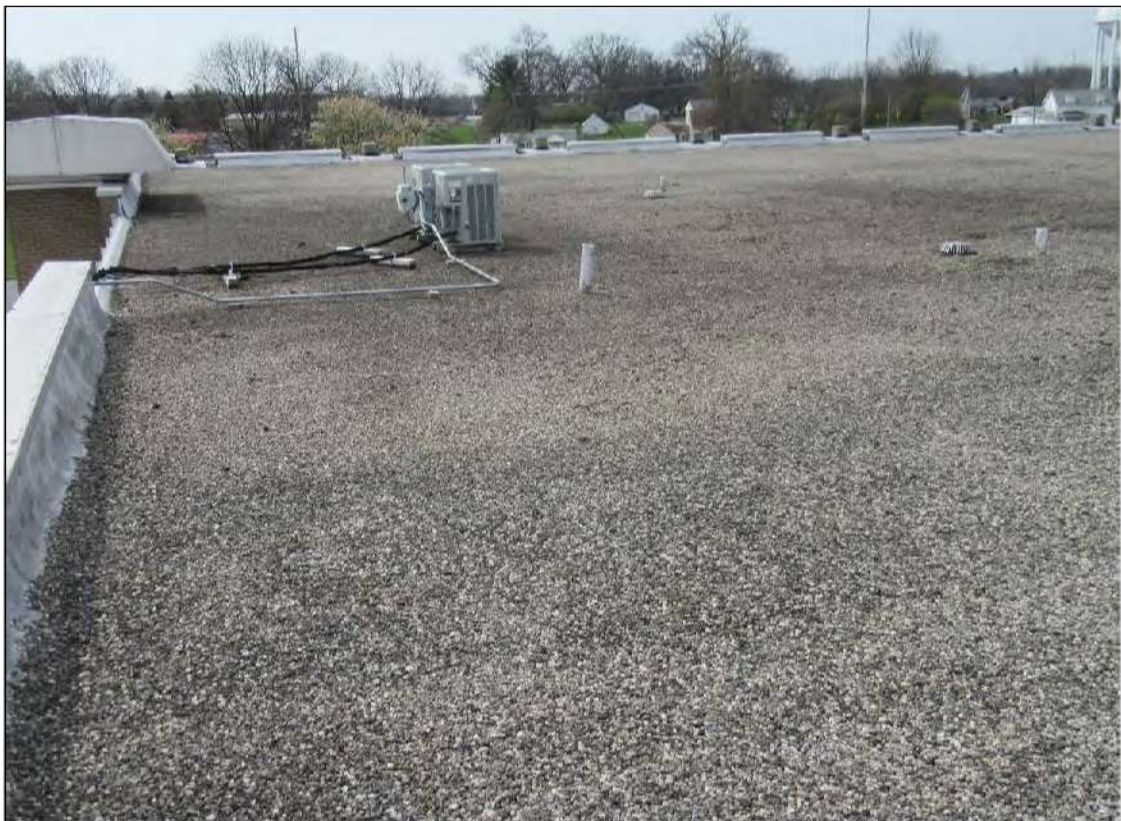
PHOTO #26: Overall view of the east edge of the roof area looking south.
