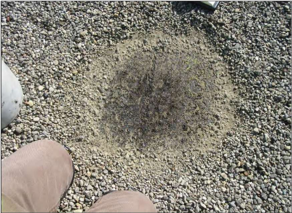
PHOTO #15: Core Cut #8 – View of Core Cut #8 location field of the roof.
