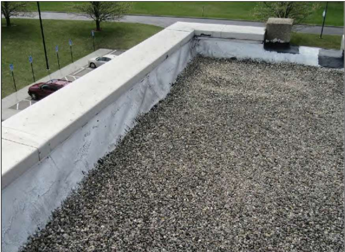
PHOTO #32: View of delaminating, sagging and wrinkled parapet wall flashing.
