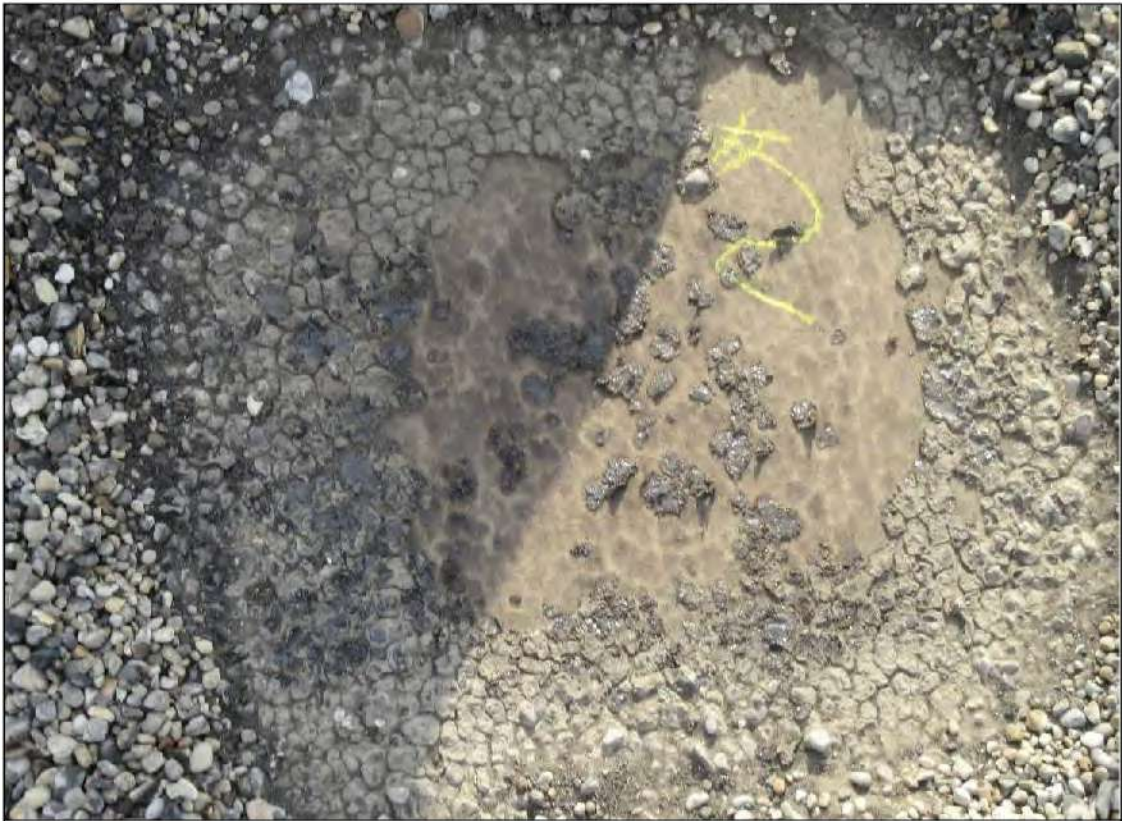
PHOTO #3: Core Cut #2 – View of Core Cut #2 located in the field of the roof between a roof drain and parapet wall.
