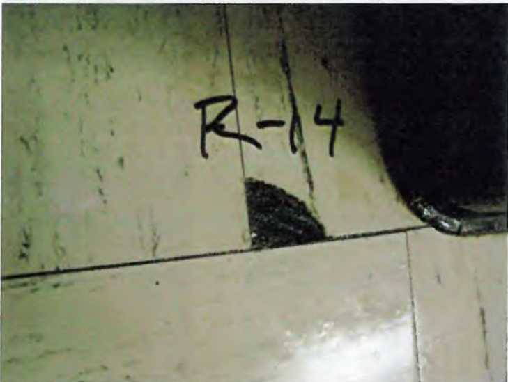
Photo 15: Off-White Floor Tile (R-14) Room 232. 2% Chrysotile Asbestos Detected (.75% Point Count). Off-White Floor Tile Mastic, 7% Chrysotile Asbestos Detected.
