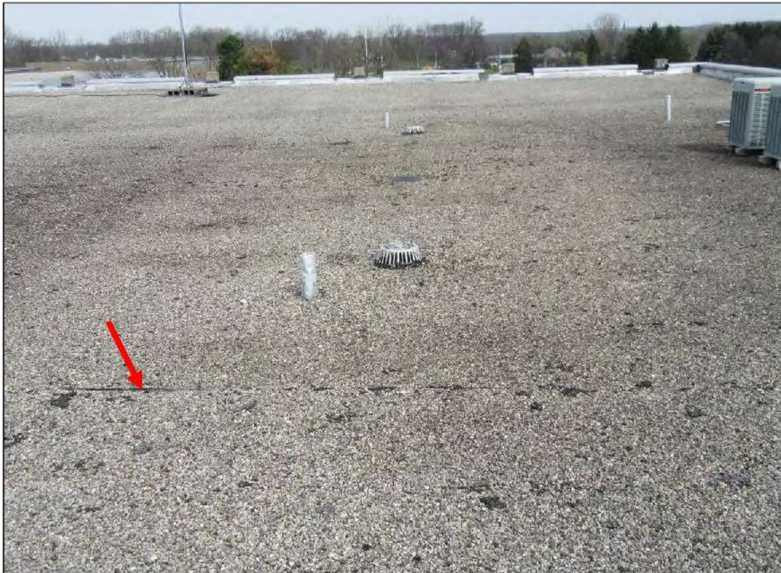
PHOTO #35: View of curling BUR membrane seams (arrow) and BUR debris spread throughout the roof area.
