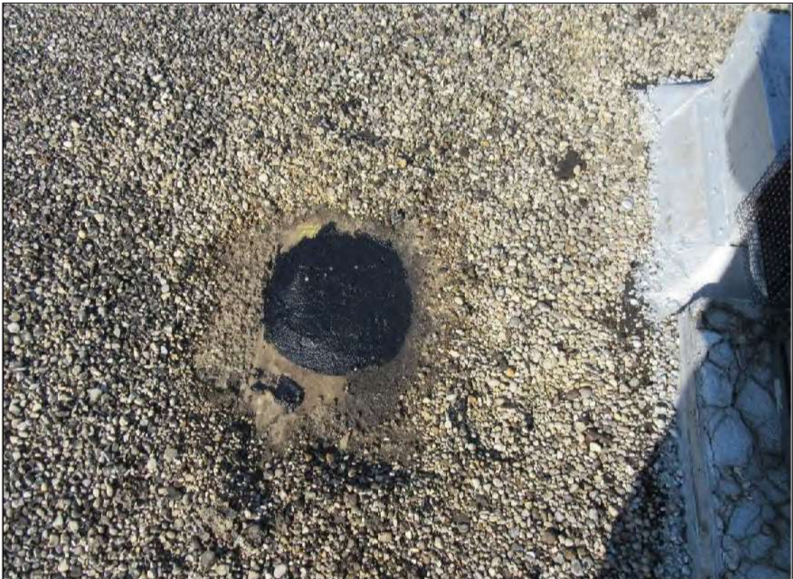
PHOTO #10: Core Cut #5 – View of roof core material, 3/4" BUR, 1/2" perlite board and 1 3/4" ISO insulation board.
