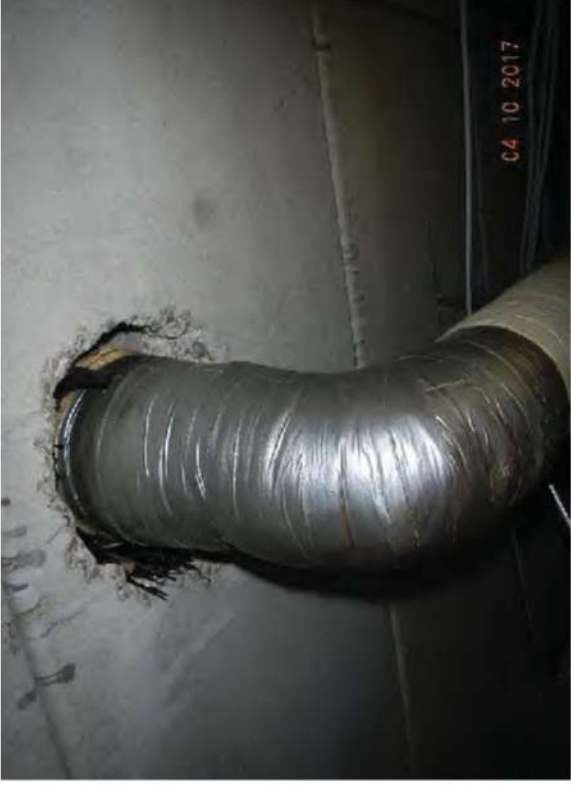
Photo 14 – View of a roof drain pipe wrapped in fiberglass insulation.
