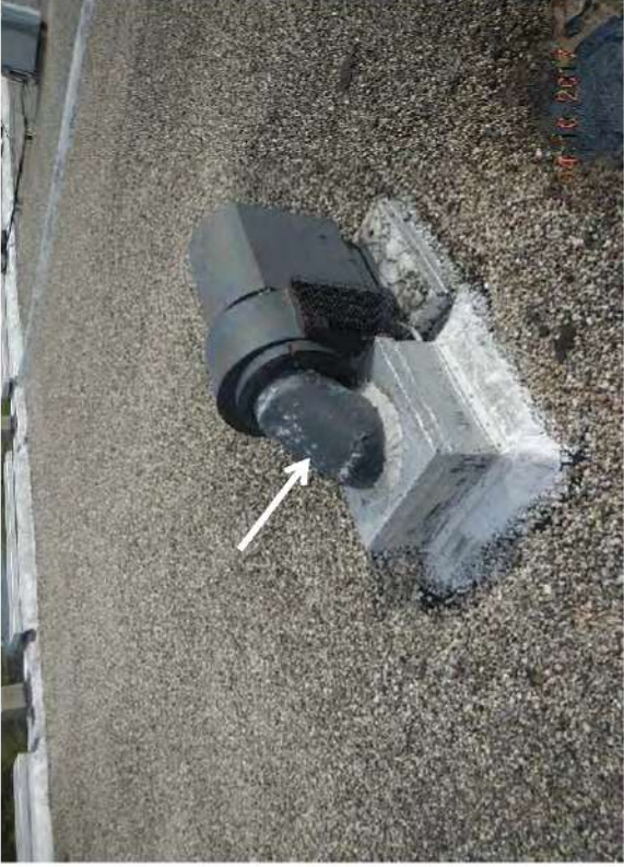
Photo 9 – View of Homogeneous Sampling Area #5, asbestos-containing gray cement exhaust duct.
