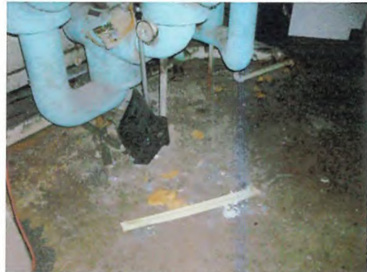
Photo 14: Elbow Mud Debris. No Asbestos Detected.
