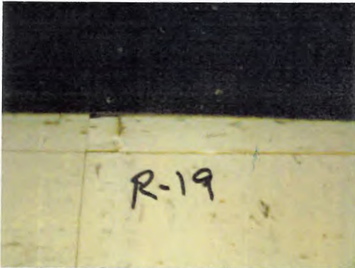
Photo 19: Off-White Floor Tile (R-19) 3 rd Floor Hallway C. 3% Chrysotile Asbestos Detected (1.75% Point Count). Off-White Floor Tile Mastic, 8.25% Point Count).
