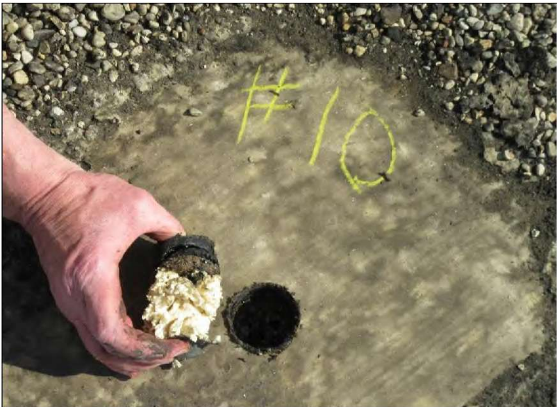
PHOTO #20: Core Cut #10 – View of roof core material 1" BUR, 1/2" perlite board (WET), 2" ISO insulation board (WET).
