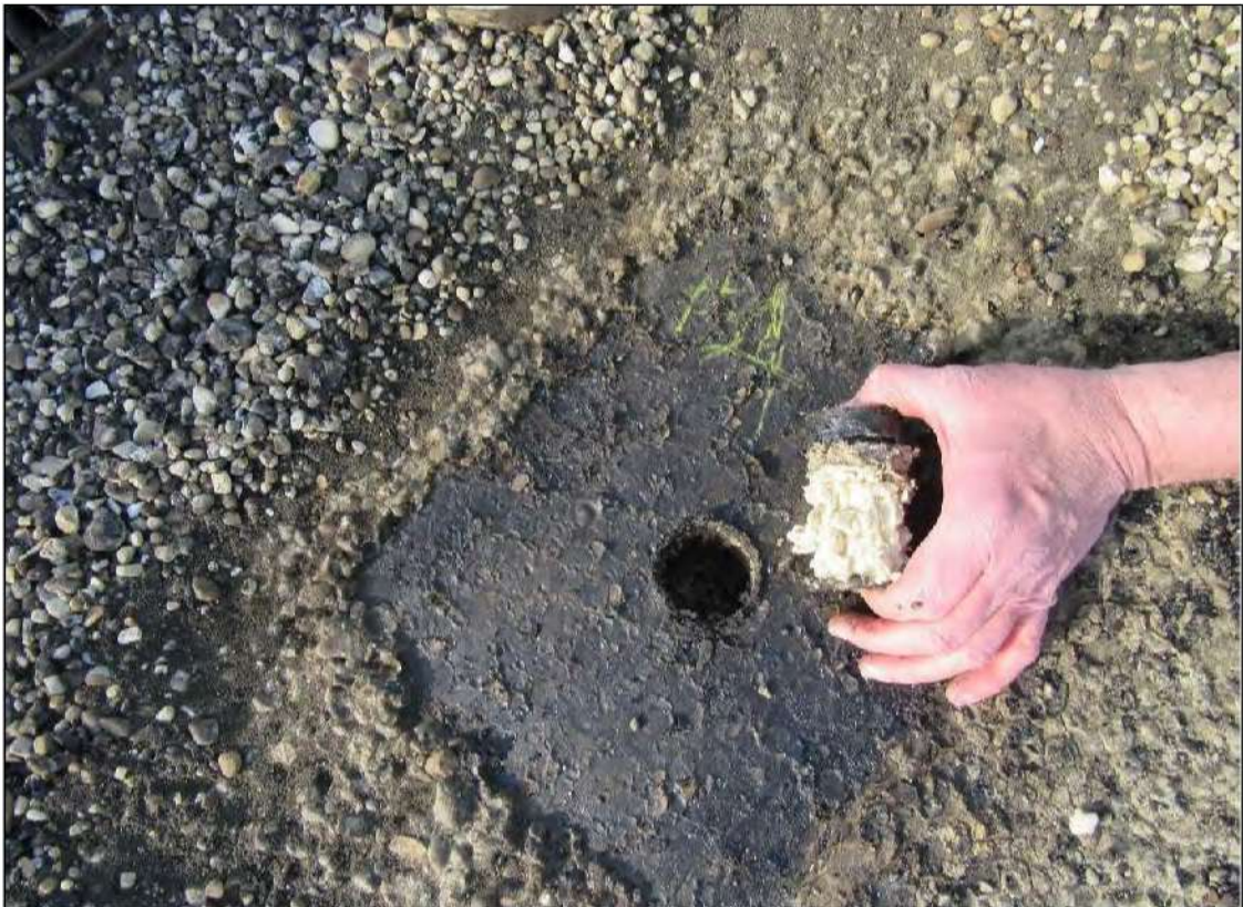
PHOTO #8: Core Cut #4 – View of roof core material, 1" BUR, 1/2" perlite board and 1 3/4" ISO insulation board.
