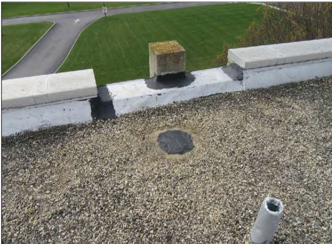
PHOTO #34: View of multiple roof cement repairs installed at the ends of coping caps and concrete pier.
