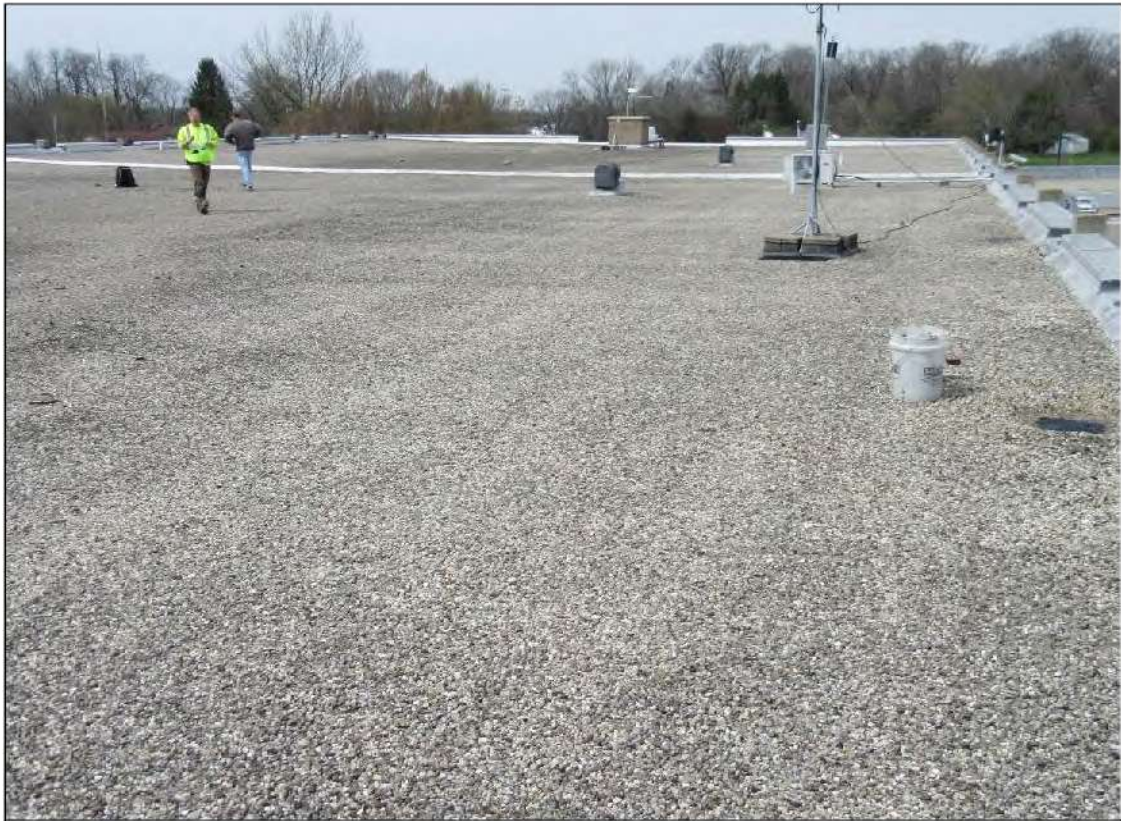
PHOTO #25: Overall view of the north edge of the roof area looking west.
