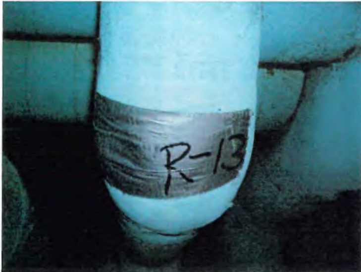
Photo 13: Elbow Mud (R-13) Fan Room. No Asbestos Detected.
