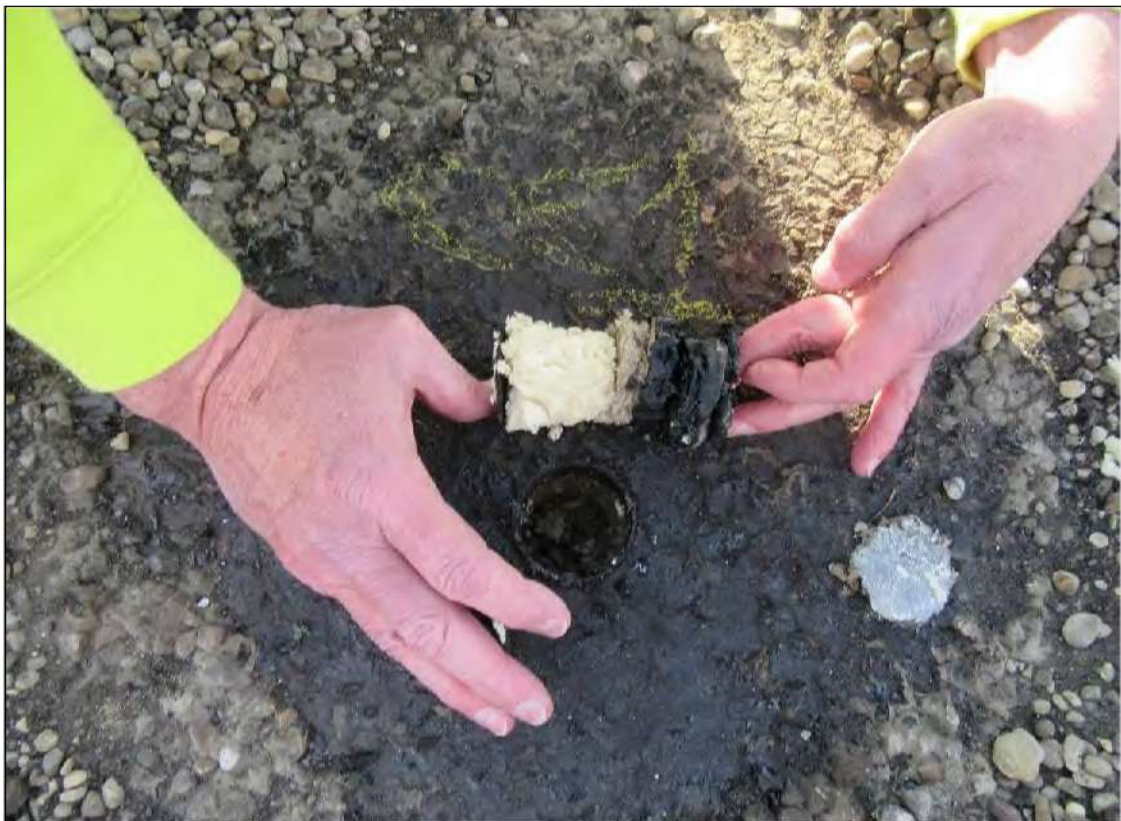
PHOTO #2: Core Cut #1 – View of roof core material, 1 1/4" BUR, 1/2" perlite board and 1 3/4" ISO insulation board.
