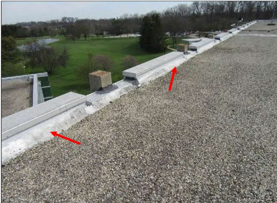
PHOTO #33: View of delaminated and bridging (arrows) parapet wall flashings. The bridging extends the length of the parapet wall.
