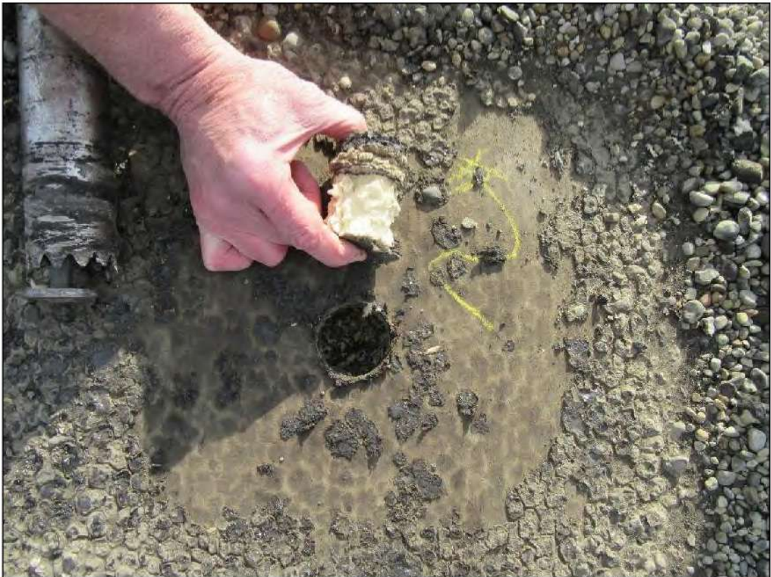
PHOTO #4: Core Cut #2 – View of roof core material, 1/2" BUR, 1/2" perlite board and 1 3/4" ISO insulation board.
