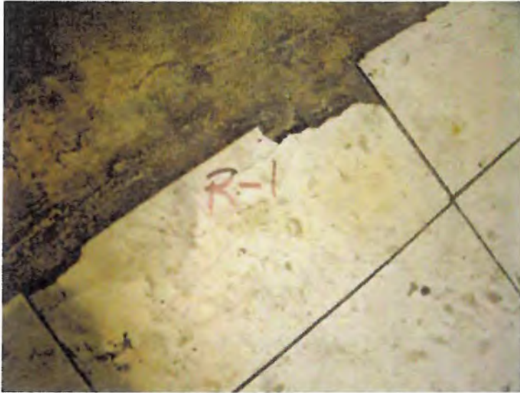
Photo 1: Off White Floor Tile (R-1) Room 106. 3% Chrysotile Asbestos Detected (2.25% Point Count). Floor Tile Mastic is 4% Chrysotile Asbestos (6.75% Point Count).
