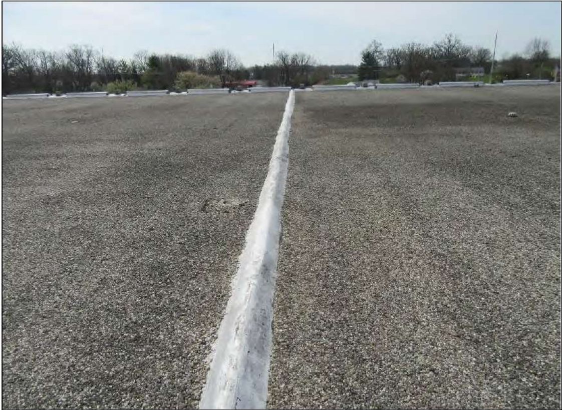
PHOTO #31: View of roof expansion joint that transverses the width of the roof.
