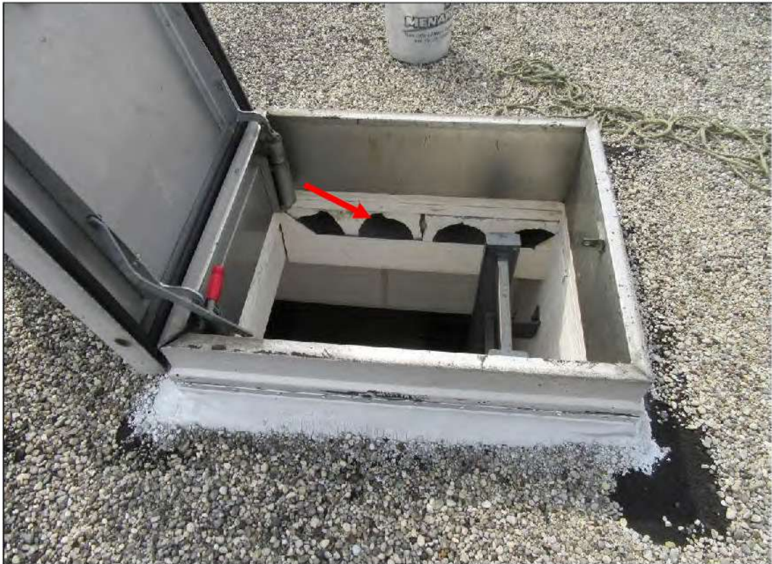
PHOTO #29: View of the precast hollow core concrete roof deck (arrow) at the roof hatch location.
