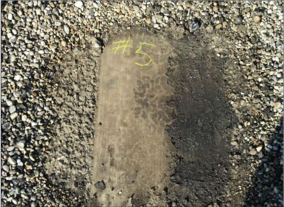
PHOTO #9: Core Cut #5 – View of Core Cut #5 located between a roof drain and parapet wall adjacent an exhaust fan roof curb. The core cut material was found to be WET.
