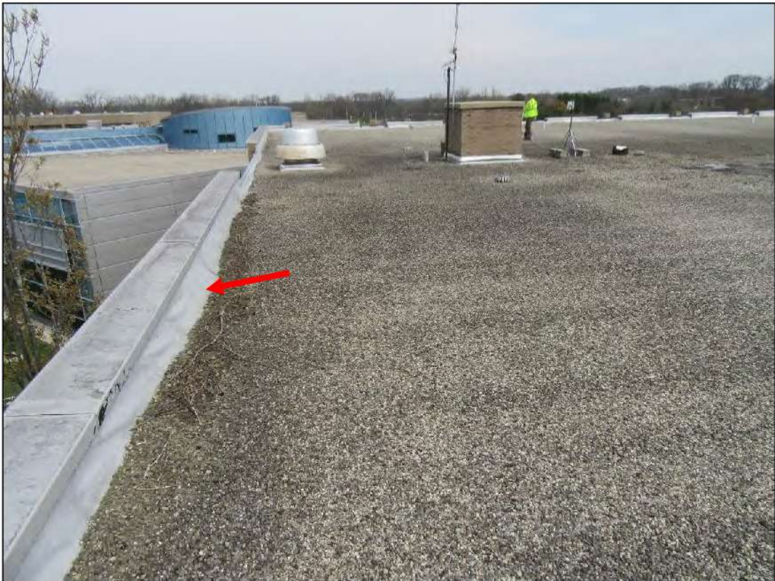
PHOTO #28: Overall view of the west edge of the roof area looking north. Note the delaminated and bridging parapet wall flashing (arrow).
