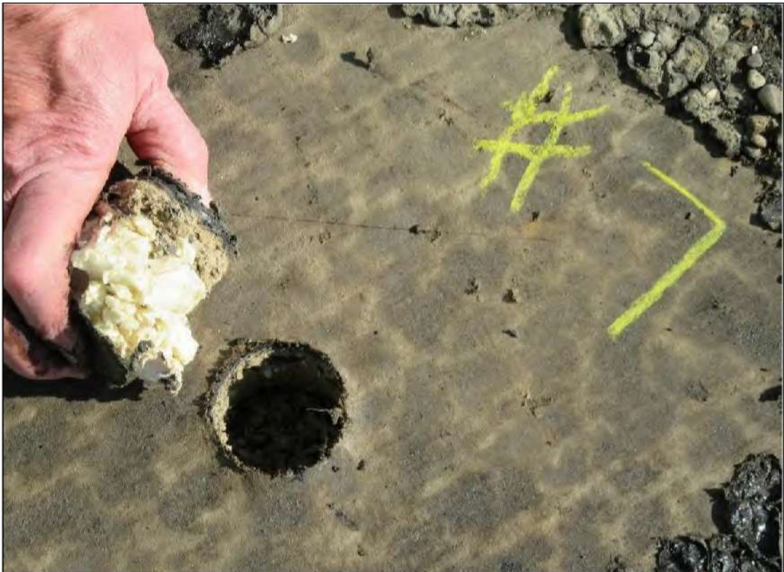
PHOTO #14: Core Cut #7 – View of roof core material 1/2" BUR, 1/2" perlite board, 2" ISO insulation board.
