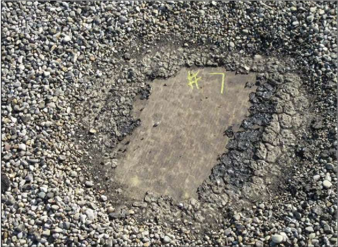
PHOTO #13: Core Cut #7 – View of Core Cut #7 location in the middle of the roof field.
