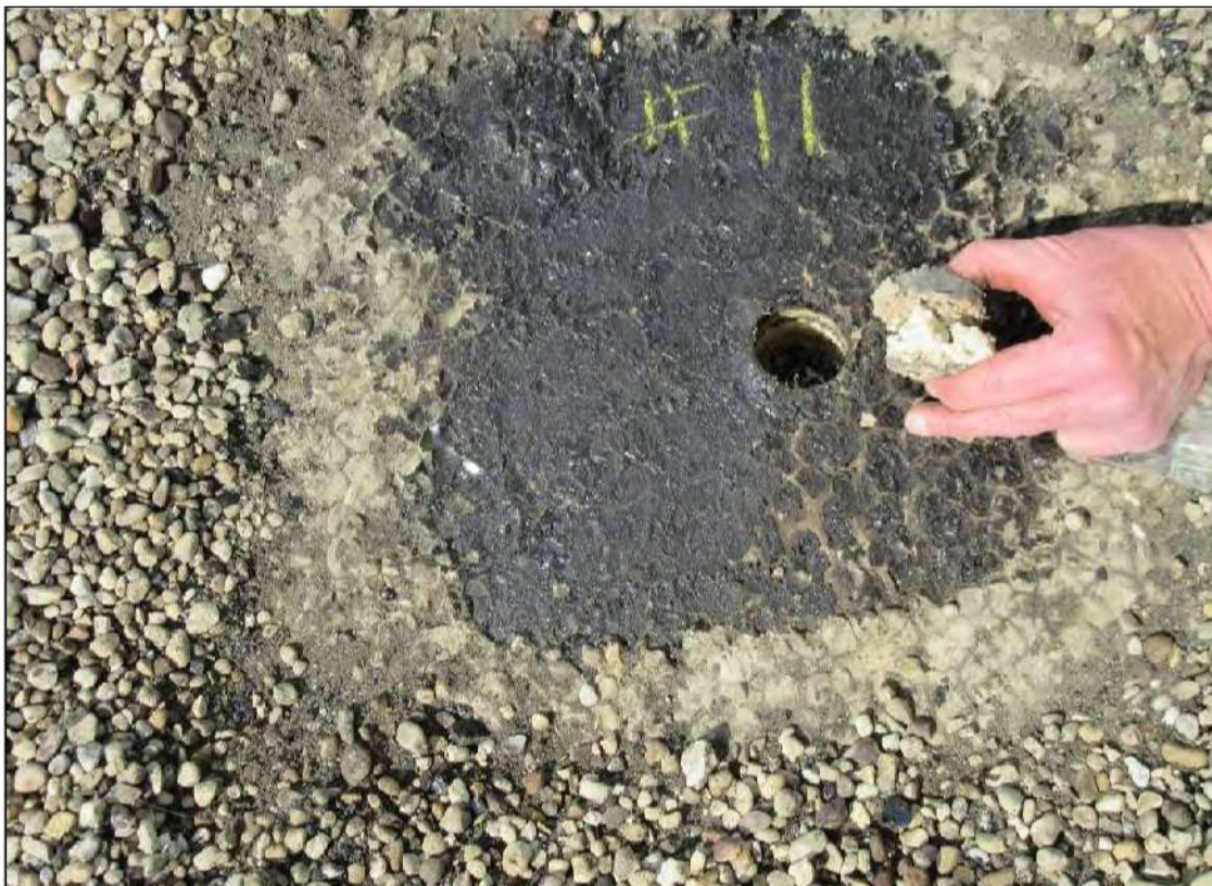
PHOTO #22: Core Cut #11 – View of roof core material 3/4" BUR, 1/2" perlite board, 2" ISO insulation board.
