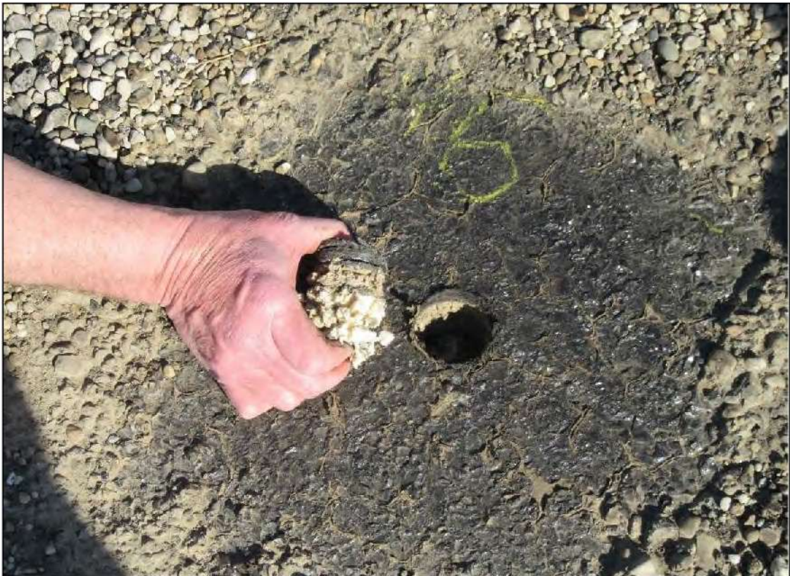
PHOTO #12: Core Cut #6 – View of roof core material, 3/4" BUR, 1/2" perlite board and 1 3/4" ISO insulation board.
