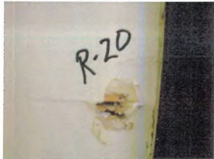
Photo 20: Drywall/JC (R-20) Room 313 Closet. <1% Chrysotile Asbestos Detected (1.50% Point Count).
