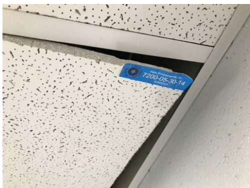
Photo 13- Sample# 7200-05-30-14, No Asbestos Detected in 2' x 4' Ceiling Tile
