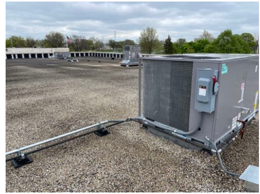
Photo 84- Electrical Insulators in Electric Safety Switches are Assumed to Contain Asbestos
