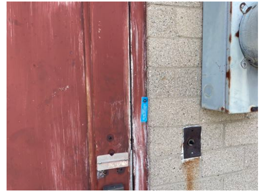
Photo 75- Sample #7277-04-16-15, 3% Chrysotile Asbestos Detected in Grey Exterior Caulk
