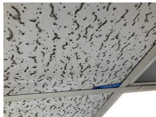
Photo 15- Sample# 7200-05-30-16, No Asbestos Detected in 2' x 4' Ceiling Tile
