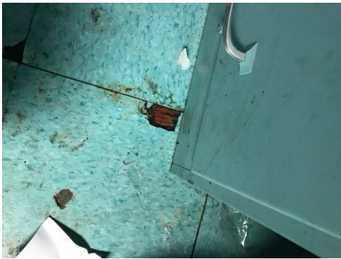
Photo 28- Confirmed 9" x 9" Asbestos Floor Tile Under Most of the Floors in the Building
