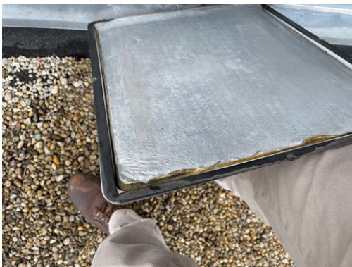
Photo 88- Rooftop Air Handler, Inside Fiberglass Insulation
