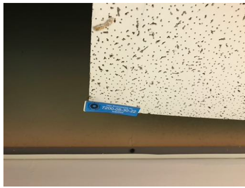
Photo 20- Sample# 7200-05-30-22, No Asbestos Detected in 2' x 4' Ceiling Tile
