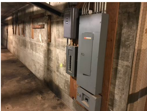
Photo 31- Basement, NE Hallway, West Wall, North Central Area, All Electrical Insulators are Assumed to Contain Asbestos
