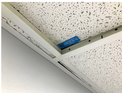
Photo 14- Sample# 7200-05-30-15, No Asbestos Detected in 2' x 4' Ceiling Tile
