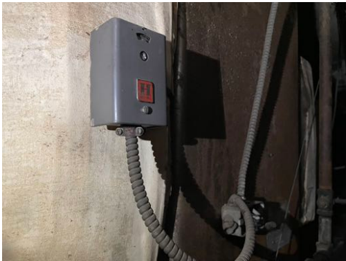
Photo 85- Electrical Insulators in Electric Safety Switches are Assumed to Contain Asbestos
