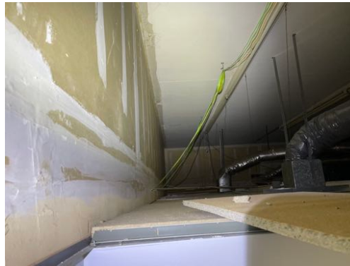
Photo 59- Sample# 7277-04-05-23, 0.25% Chrysotile Asbestos in Joint Compound, No Asbestos in Drywall
