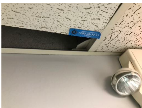
Photo 16- Sample# 7200-05-30-17, No Asbestos Detected in 2' x 4' Ceiling Tile
