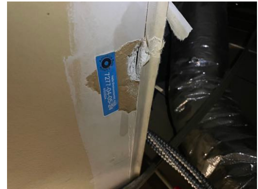
Photo 60- Sample# 7277-04-05-24, 0.5% Chrysotile Asbestos in Joint Compound, No Asbestos in Drywall
