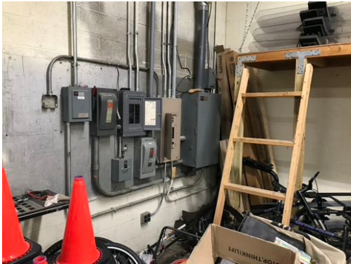
Photo 32- 1st Floor, Bicycle Garage, North Wall, NE Corner, All Electrical Insulators are Assumed to Contain Asbestos
