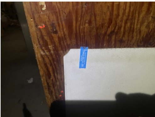
Photo 119 - Sample 7462-03-31-29 with 15% asbestos
