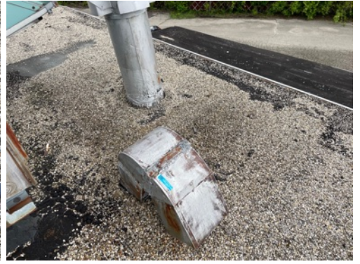
Photo 144 - Sample 7462-04-30-05 with 3% asbestos
