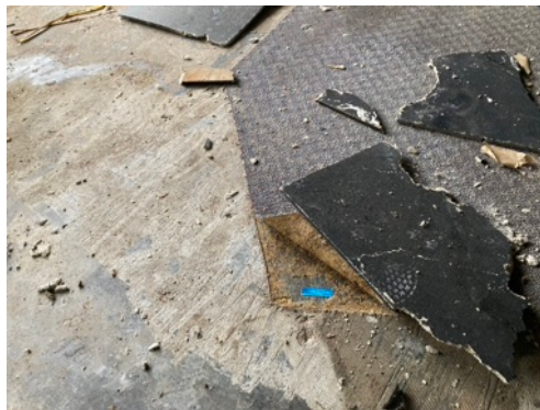
Photo 89 - Sample 7462-03-18-45 with 2% asbestos
