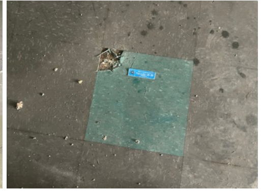
Photo 84 - Sample 7462-03-18-39, 3% Asbestos in mastic only
