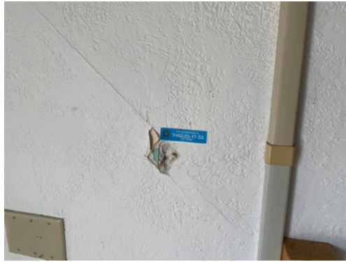
Photo 41 - Sample 7462-03-17-53, <1% Asbestos in Texture only
