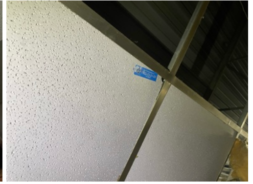
Photo 97 - Sample 7462-03-31-03 with <1% amosite asbestos
