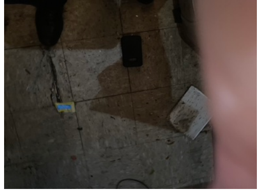
Photo 109 - Sample 7462-03-31-16 with 2% asbestos in tile and 3% asbestos in mastic
