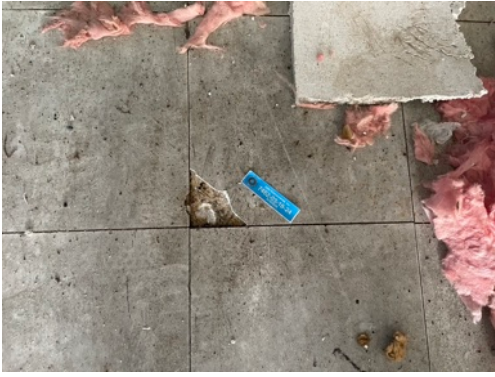
Photo 73 - Sample 7462-03-18-24, 3% Asbestos in mastic only
