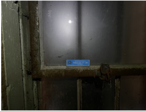
Photo 32 - Sample 7462-03-17-38, <1% Asbestos Detected
