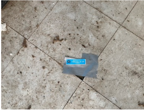
Photo 74 - Sample 7462-03-18-25, 3% Asbestos in mastic only
