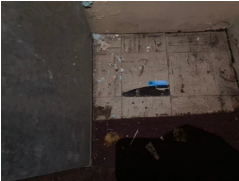
Photo 43 - Sample 7462-03-17-55 with 5% asbestos in tile and 3% asbestos in mastic
