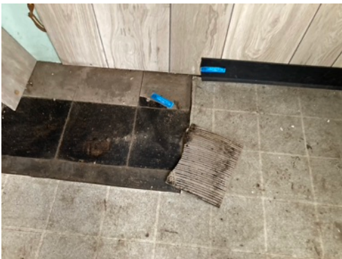
Photo 25 - Samples 7462-03-17-28, -29, 4% Asbestos Detected in tile only
