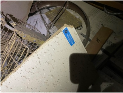
Photo 98 - Sample 7462-03-31-04 with <1% amosite asbestos
