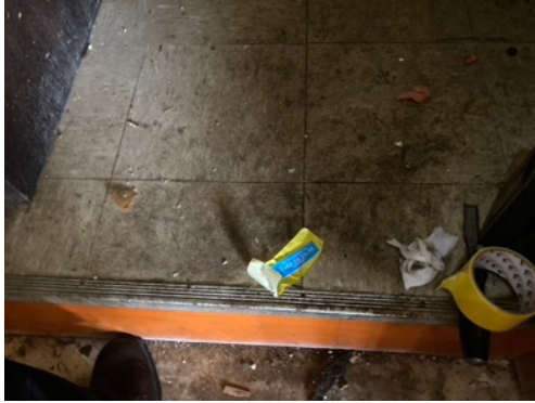
Photo 108 - Sample 7462-03-31-15 with 2% asbestos in tile and 3% asbestos in mastic
