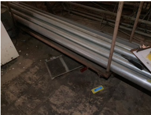
Photo 107 - Sample 7462-03-31-14 with 3% asbestos
