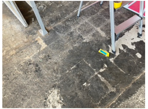
Photo 106 - Sample 7462-03-31-13 with 3% asbestos
