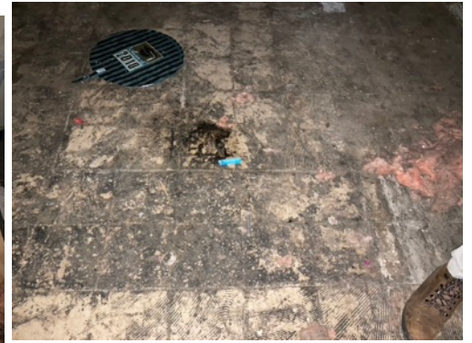
Photo 124 - Sample 7462-03-31-36 with 2% asbestos in tile and 3% asbestos in mastic
