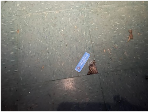
Photo 85 - Sample 7462-03-18-40, 3% Asbestos in mastic only
