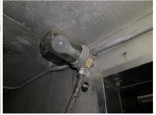
Photo 93 - Explosion-proof light in cooler assumed to contain asbestos
