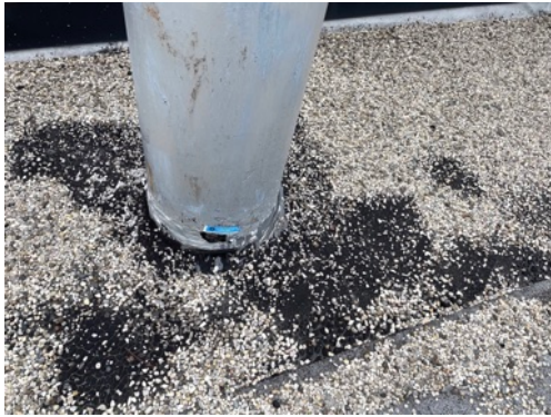
Photo 145 - Sample 7462-04-30-06 with 3% asbestos
