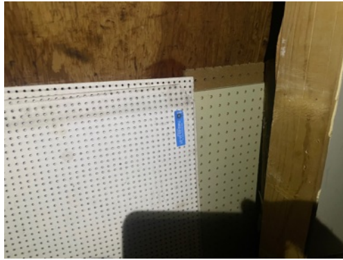
Photo 117 - Sample 7462-03-31-27 with 15% asbestos
