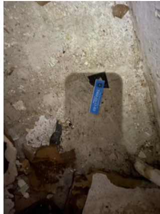
Photo 50 - Sample 7462-03-17-63, 3% Asbestos in mastic only
