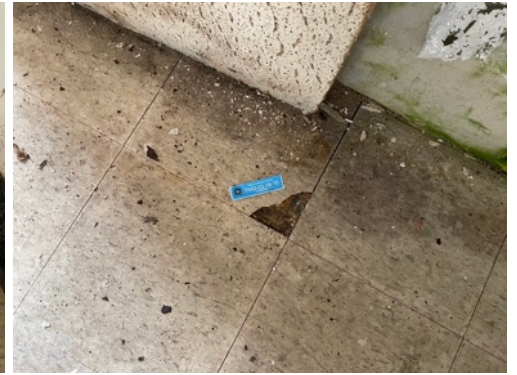
Photo 60 - Sample 7462-03-18-10, 3% Asbestos in mastic only
